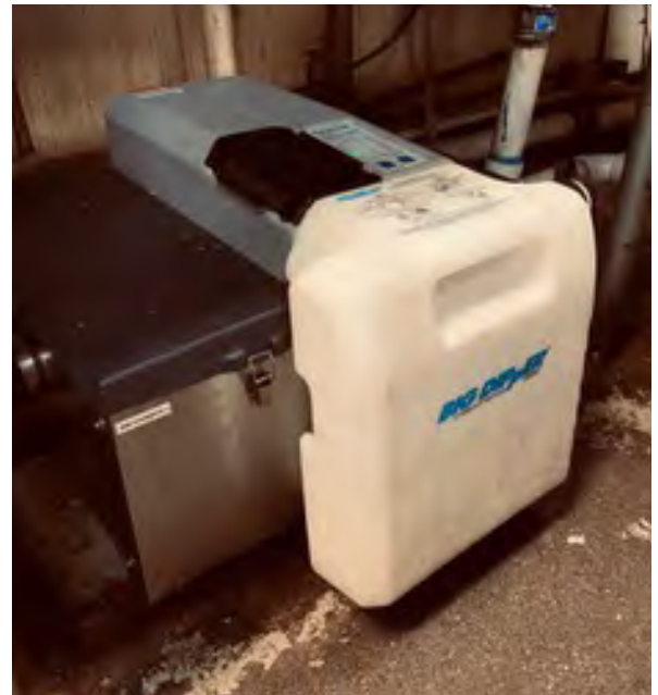
Big Dipper, W-200-IS, installed at Life's Kitchen
