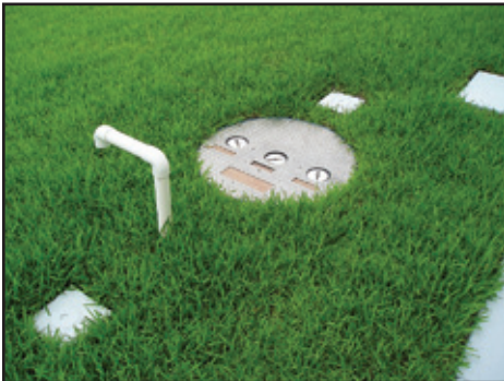
TZ-600 Installed in Green Space outside of Restaurant
