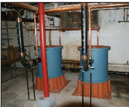
Two TZ-600 Units Servicing Correctional Facility in NE United States
