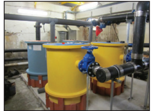
Two Solids Separators and two Grease Interceptors handling the flow from the food court in a large shopping mall.
